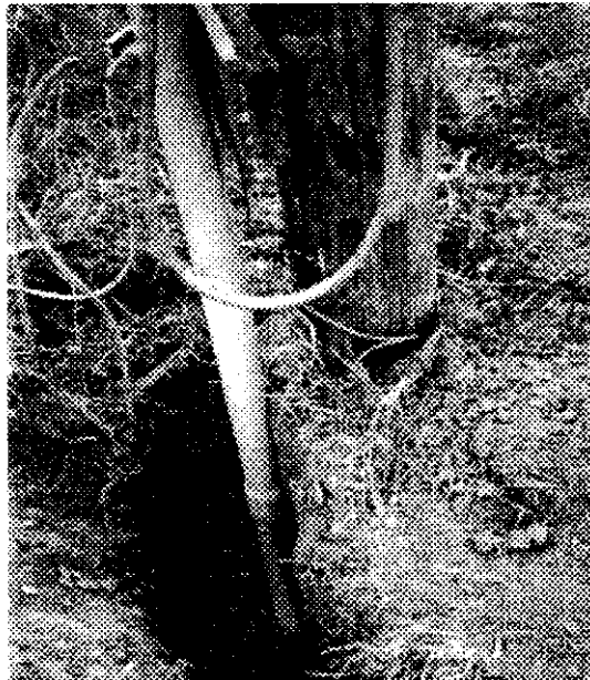
The new electrical feed is run underground above the water line from this pole to the house.
