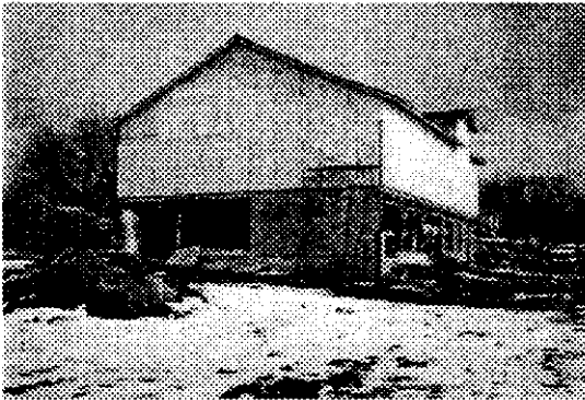
View of the soon-to-be residence from the southwest. The upper two levels have been enclosed with insulation on the exterior.
